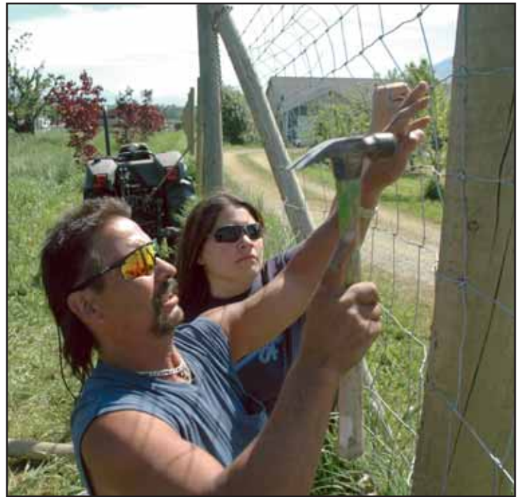
Alan Cortez and Amanda Shelton of the Tulalip Tribes nail a length of fence into place. Photo: J. Shaw
