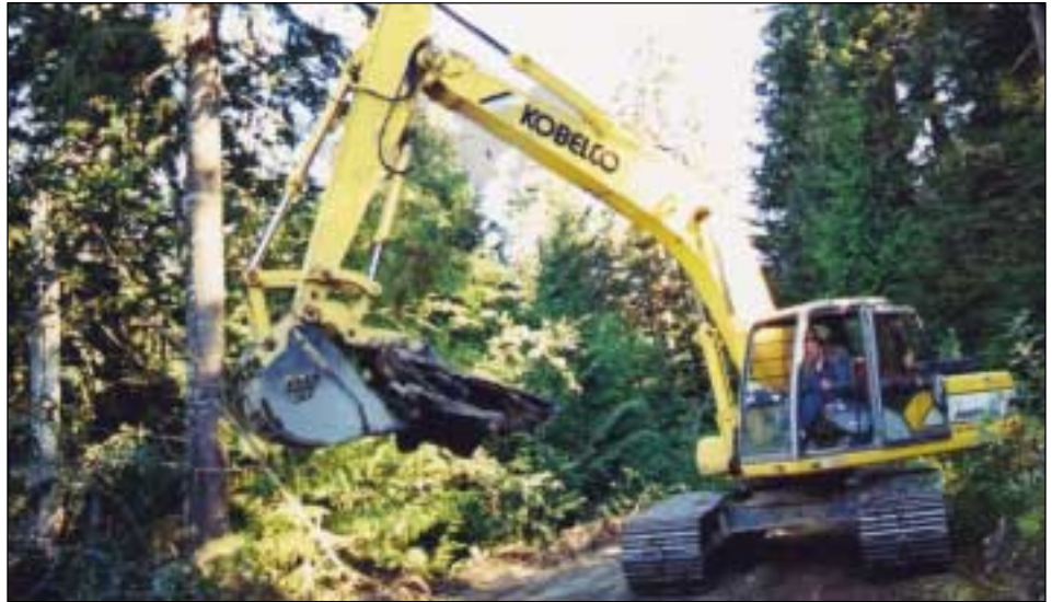
Road decommissioning and upgrade work by the Skagit River System Cooperative, such as removal of failing culverts, will help prevent catastrophic landslides that are harmful to fish habitat. Photo: J. Shaw
