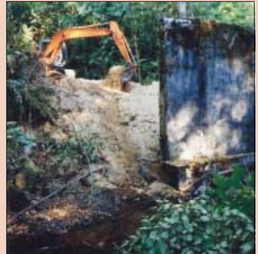
The Stillaguamish Tribe removed tons of concrete, wood and metal left by a collapsed bridge, opening miles of upstream fish habitat. Photo: J. Shaw
