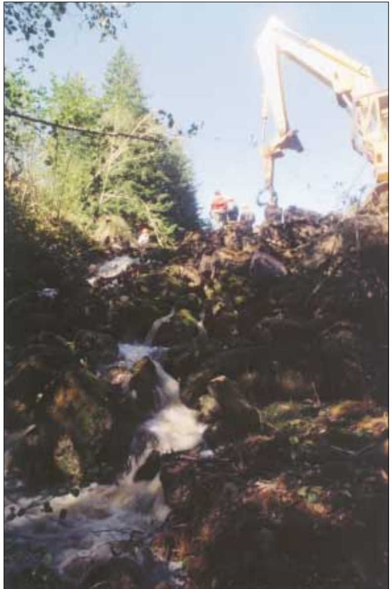
The Makah Tribe removed a 25-foot dam on Wa'atch Creek to improve fish habitat. Photo: D. Preston
